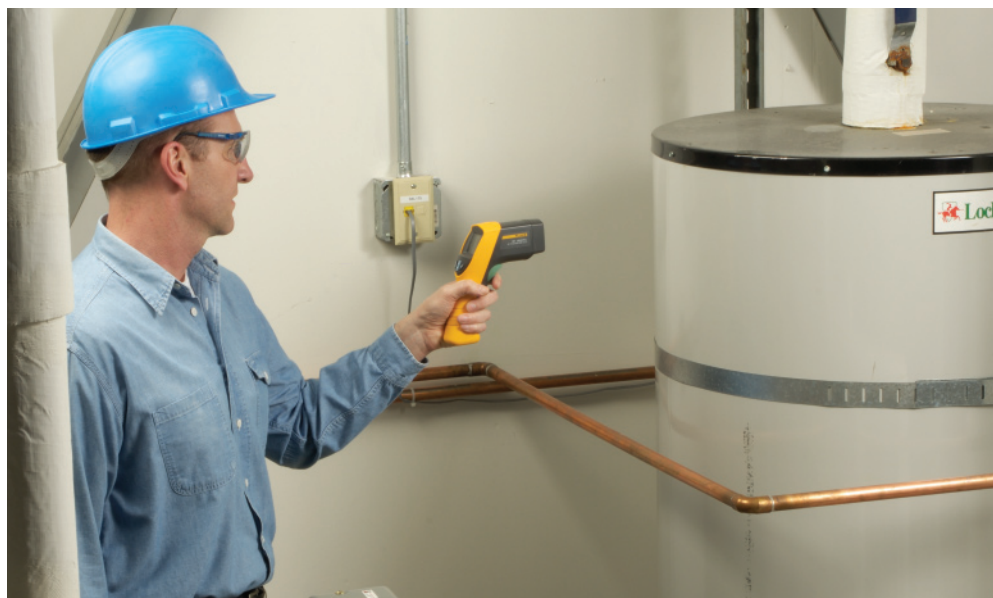
A quick infrared survey can check for leaks and uneven temperatures in both the heater and pipes.
