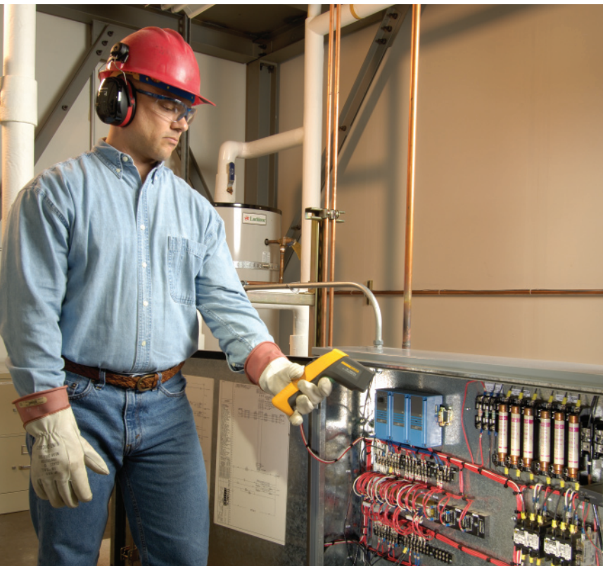
Measuring temperature of fuses and electrical connections.
